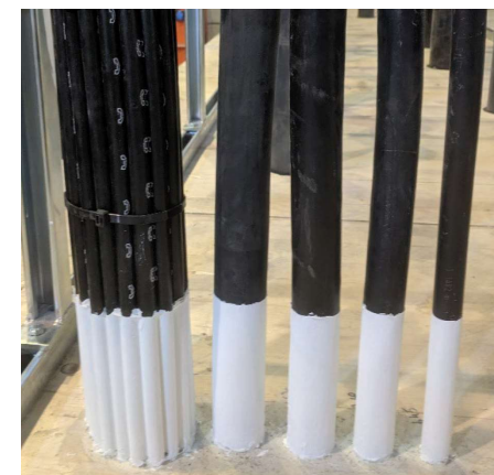
Typical sample of penetrating services with annular gap widths between 10 and 20mm
